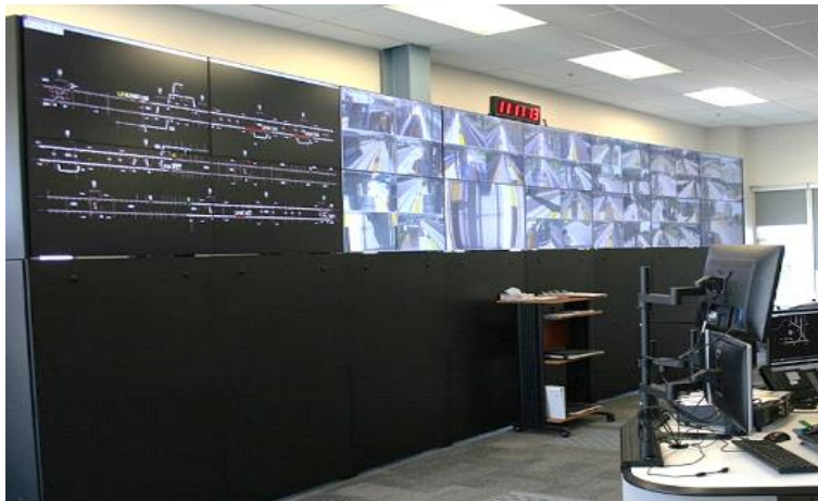
Figure 5.1 Typical Operations Control Room
